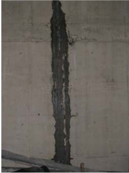
Leak through joints in concrete wall. Water is 'running' therefore exceeds 'some seepage' criterion.
