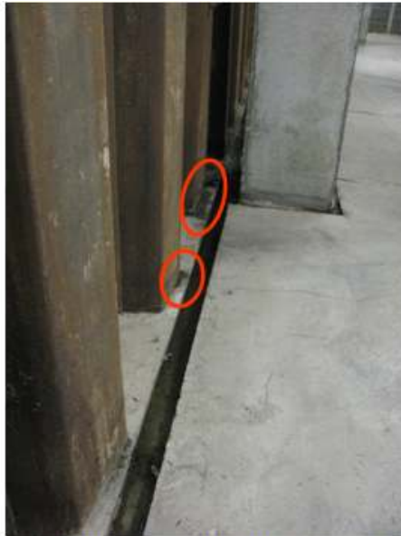
Grade 1 internal environment. Damp patches on slab. Traces of water in channel on floor.
