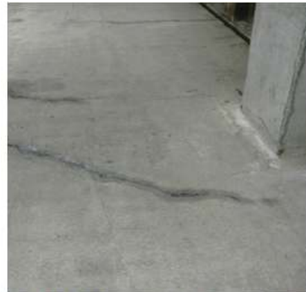
Grade 1 internal environment. Some seepage and beading through cracks but water not flowing.
