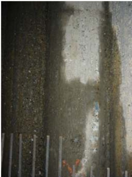
Leak through joints in secant pile wall. Water is 'running' and damp patches exceed 10% of wall face.
