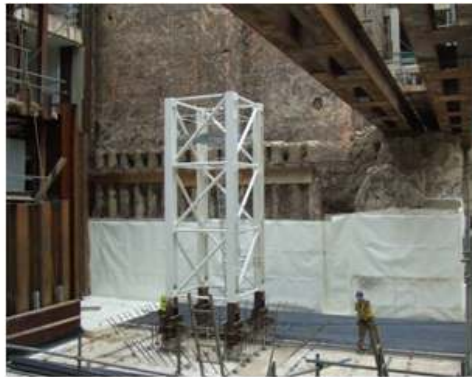
Membrane being applied to substructure walls and beneath slab. It will bond to the concrete cast against it.
