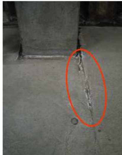
No damp patches but discolouration to slab due to evaporation of moisture.
