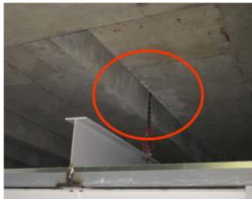
No damp patches but discolouration to concrete on underside of slab due to evaporation of moisture.
